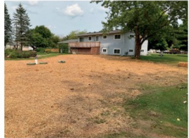
The manhole covers are left above grade for future service and maintenance. A power post equipped with a visual and audible alarm is installed to alert when there is an issue that needs attention.
